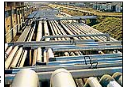
If WTS is right, natural gas pipes like these will carry broadband technology to millions of Americans in the not-too distant future.
